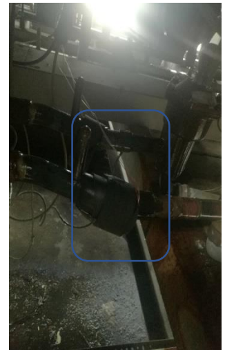
Others are all with copper pipes
